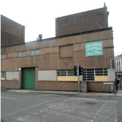
Building in poor state of repair
