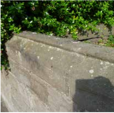
Iron work has been removed in some cases
