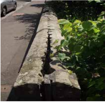
Cracked boundary wall
