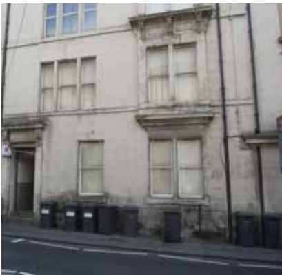
Discoloured wall surface opposite the parks main entrance
